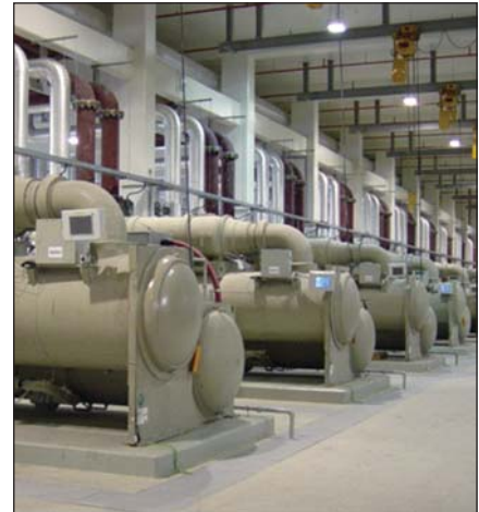
Water-cooled centrifugal chiller plant.
